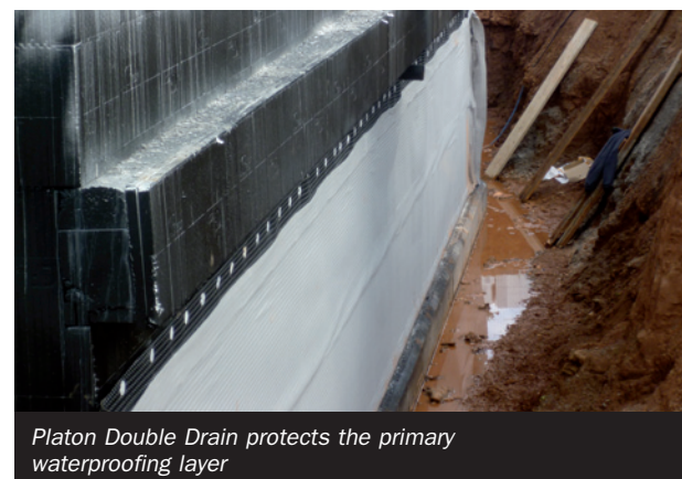
Three coats of TT Vapour Membrane were spray applied to the exterior
