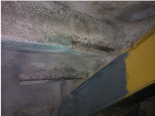
A prepared area after removal of spalled concrete and cleaning of the reinforcement
