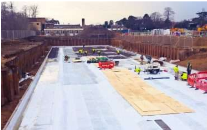
Newton 403 HydroBond was applied on this 193-apartment development by Crest Nicholson in Sunbury-on-Thames
