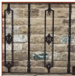
Ornate & Victorian balusters
